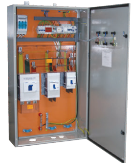
Low Voltage Main Switchboard Type GRT
